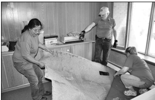
Volunteers from Lowe’s rip out old carpet from the office at 21 1/2 North Franklin Street on United Way’s Community Care Day 2009. The refurbishing paved the way for the opening of the North Star Center.
